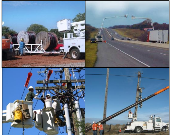
TSEC Power Distribution Services
